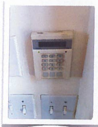
Obsolete & non-functional alarm system
