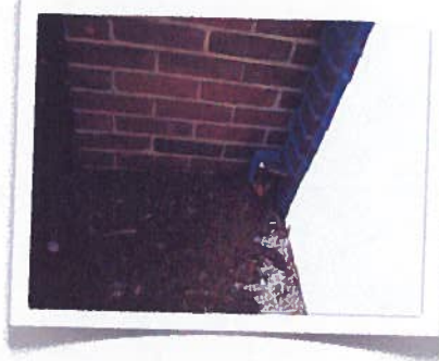
Electrical box damage
