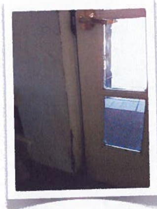
Loose door latch & door area kick damage
