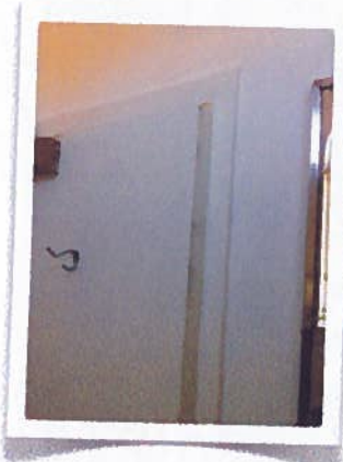
Bathroom door off hinges
