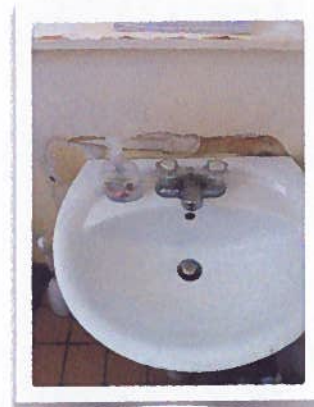
Water damage, counter chipping, & non-ADA sink
