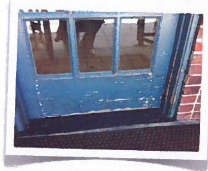
Exterior kick & paint damage (door, door frame, & window frames)
