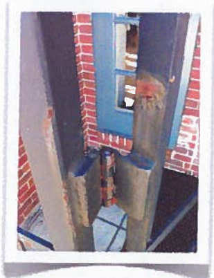
Exterior rust & paint damage (wrought iron gate)
