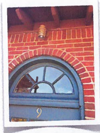
Exterior lights not functioning (over door & windows)
