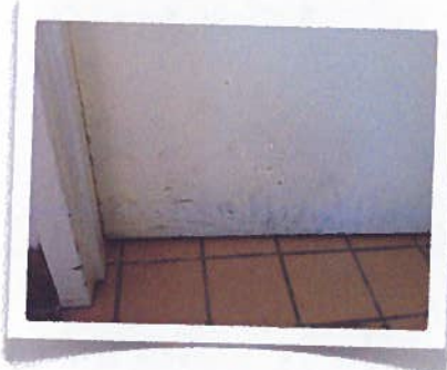
Kick damage on bathroom doors
